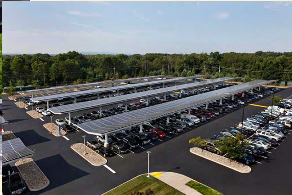
Solar @ Worcester Business Center
