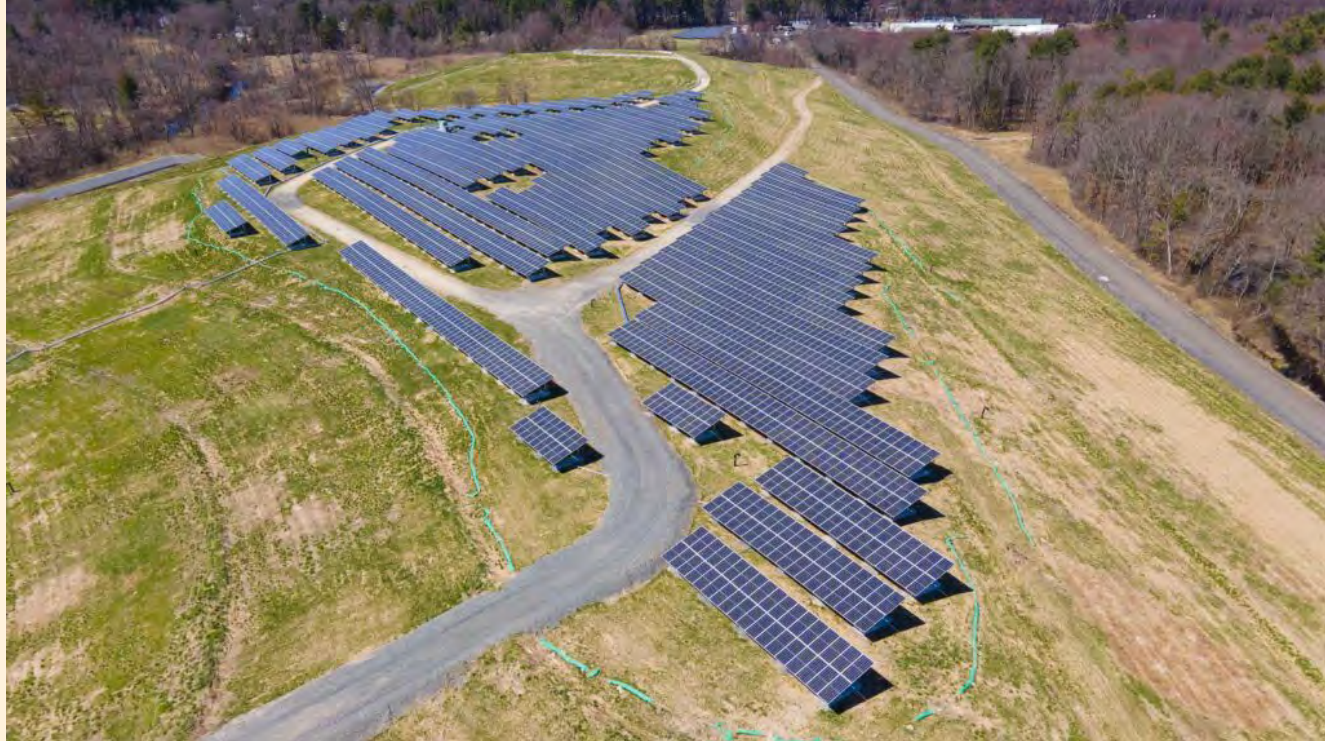
Solar @ Landfill in Tewksbury
