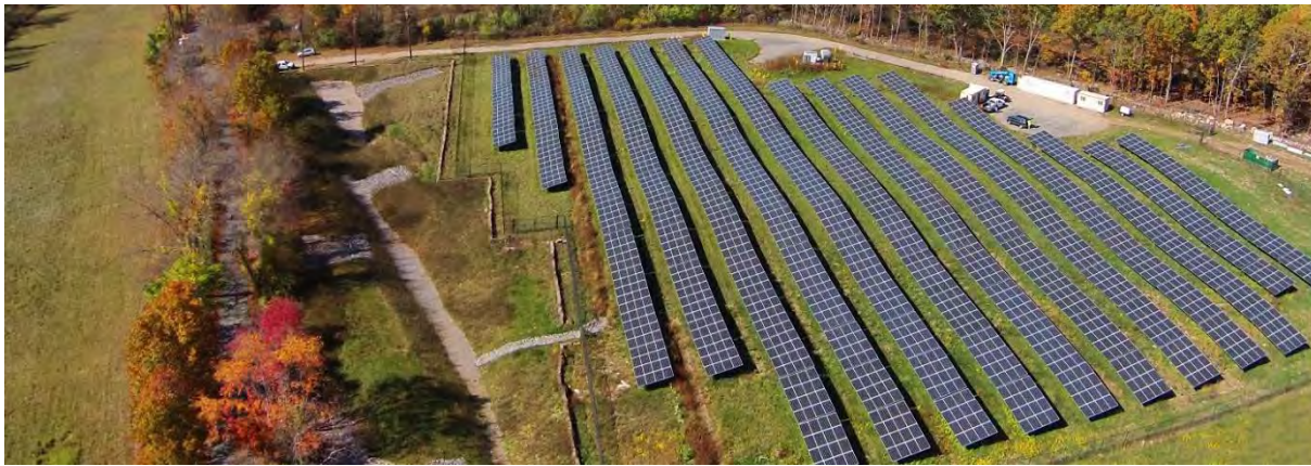
BlueWave Capital solar array, Grafton MA
